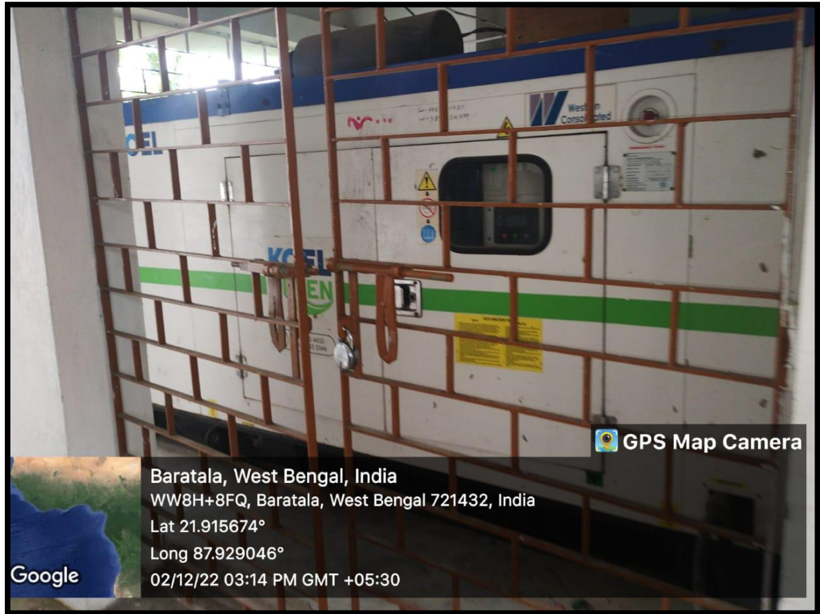
Digital Generator within Campus
